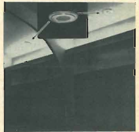
Ceiling speakers are installed in church where this amplifier is used.
