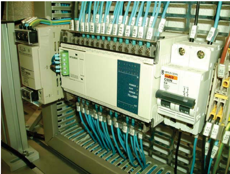
Fig.1.1. A typical industrial PLC
