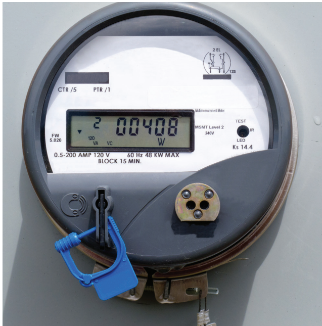
Figure 3.14 An example of a smart electricity meter.
