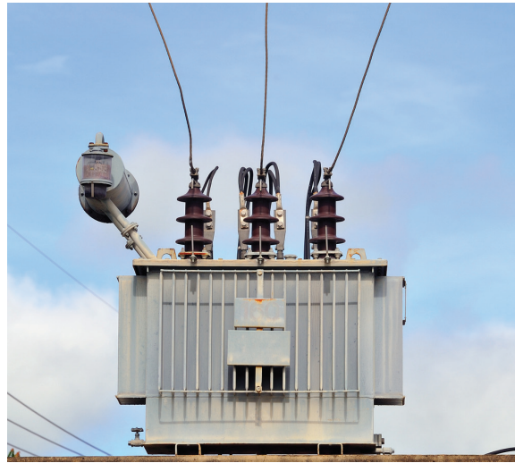
Figure 2.56 A 3ph transformer.
