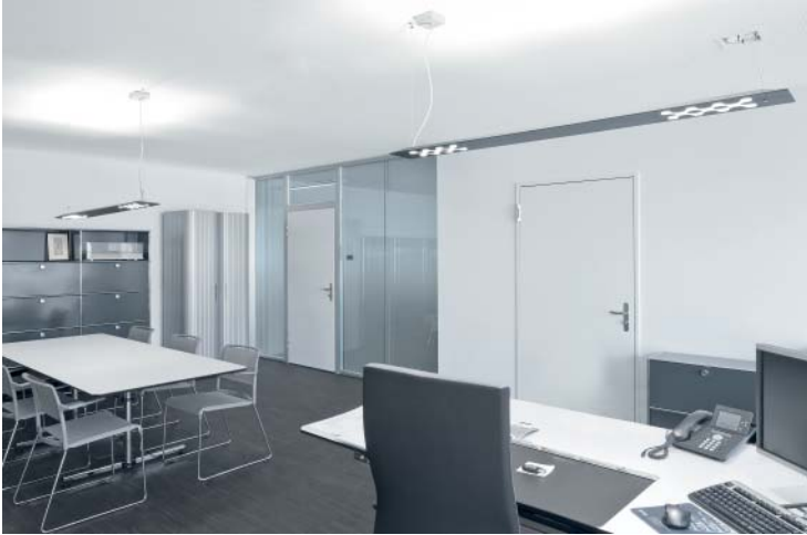
Figure 7.7 An office LED luminaire with direct and indirect light contributions on the ceiling. (Reproduced with permission from Trilux (Arnsberg, Germany).)
