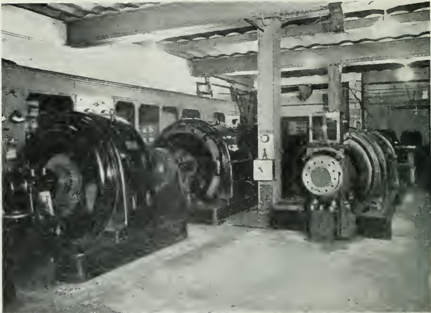
Fig. 3. 300-kW. Generator which supplies energy for the Transmitter at 500 volts and 1,000 cycles.
