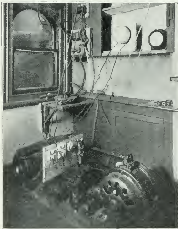
Fig. 2. The generator unit with driving motor.
