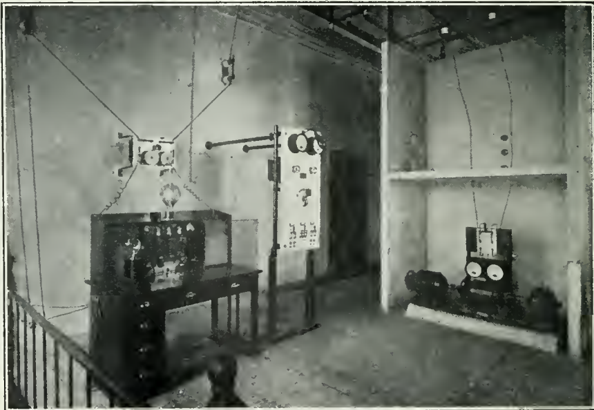
Cabinet Telephony Set as installed at a sub-station.
