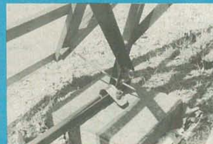
FIG. 26—CONCRETE BASE PADS support and anchor the four corners of the antenna. Anchor bolts and "J" clips secure the antenna to the pads.
