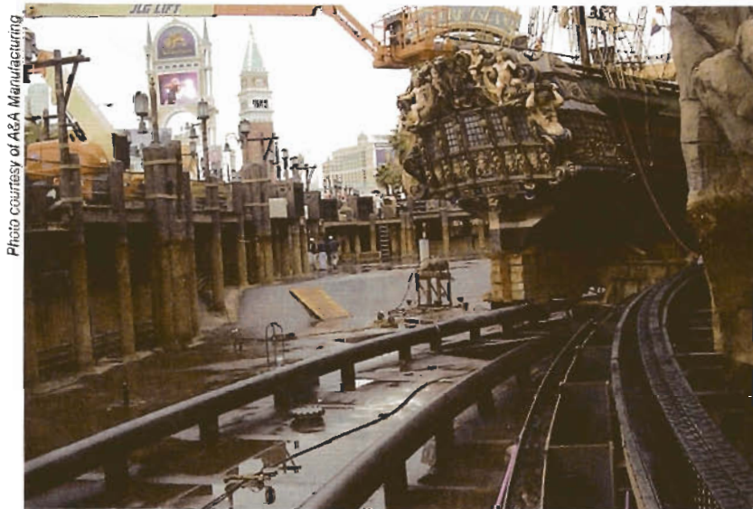
A Nylatrac cable carrier manages underwater cables that supply power to the pirate ship at Treasure Island Hotel and Casino in Las Vegas, as it moves back and forth during nightly shows.
