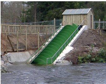
Figure 5.9 An example of an Archimedean screw at the River Dart country park, Devon. Credit: WRE Limited.
