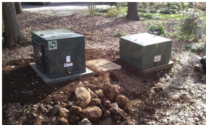
Figure 26 Community energy storage unit.
