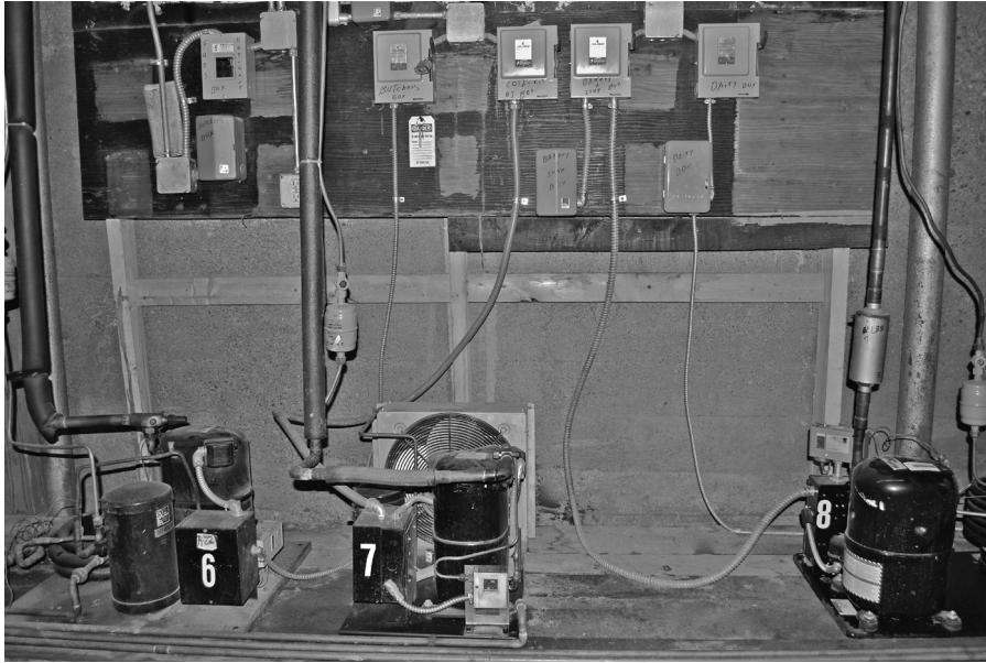
FIGURE 13-3 Three air-cooled compressors in a compressor room.
