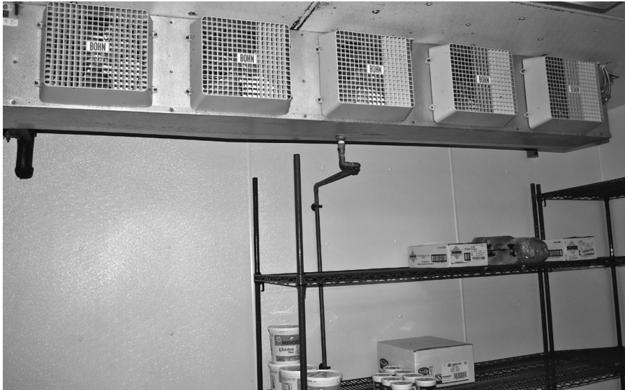
FIGURE 13-2 Five evaporators in a walk-in cooler.
