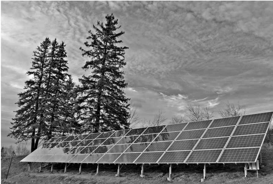
FIGURE 15-2 Solar PV array.
