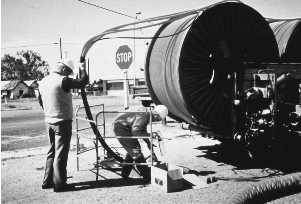
FIGURE 17-2 Long outside fiber optic runs require precision splices. (Courtesy of Fiber Optics Association.)
