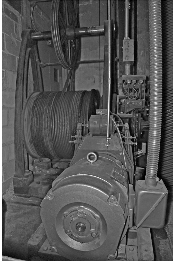
FIGURE 11-1 Elevator motor with cable drum.
