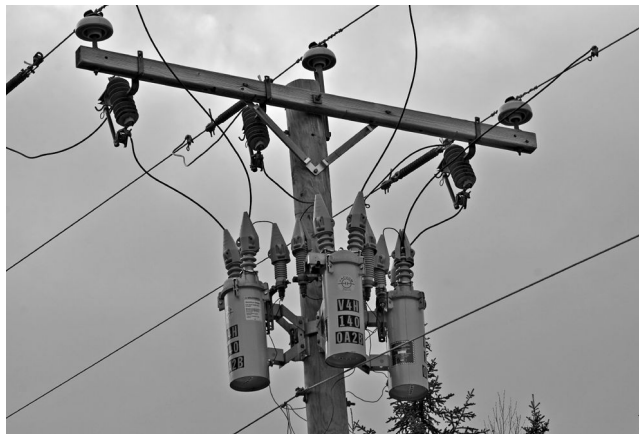
FIGURE 5-2 Three-phase transformer array.
