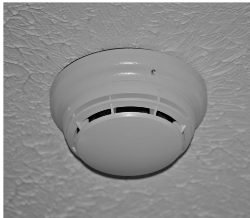
FIGURE 12-1 Smoke detector on a finished ceiling.
