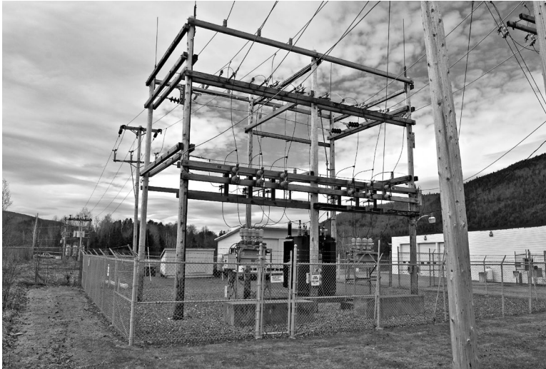
FIGURE 5-1 Substation with grounded fence.
