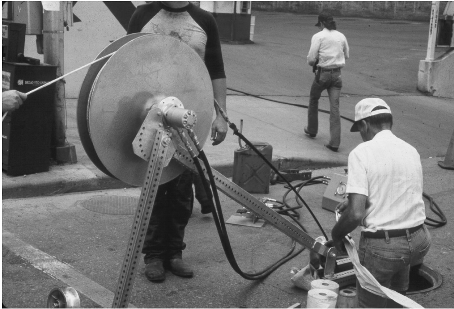
FIGURE 17-1 Outside fiber optic installation requires a large capital investment. (Courtesy of Fiber Optics Association.)
