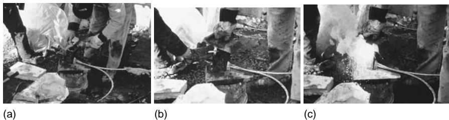
FIGURE 10.230 Exothermic bonding is the preferred method of joining the elements of a ground system. This photo sequence illustrates the procedure: (a) the powdered copper oxide and aluminum compound are added to the mold after the conductors have been mechanically joined; (b) final preparation of the bond before igniting; (c) the chemical reaction that bonds the materials together.
